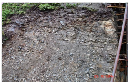
图1 嘎隆拉隧道破碎围岩地层 Fig.1 Broken rock mass of Galongla tunnel
